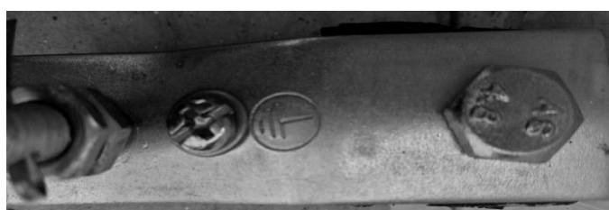
Fig. 1.24: Earthing Plate in fan
